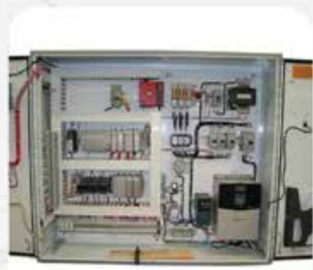
PLC Panel with VFD.
